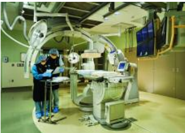
Suspended equipment keeps rooms free of obstacles like electrical cords and oxygen lines.
